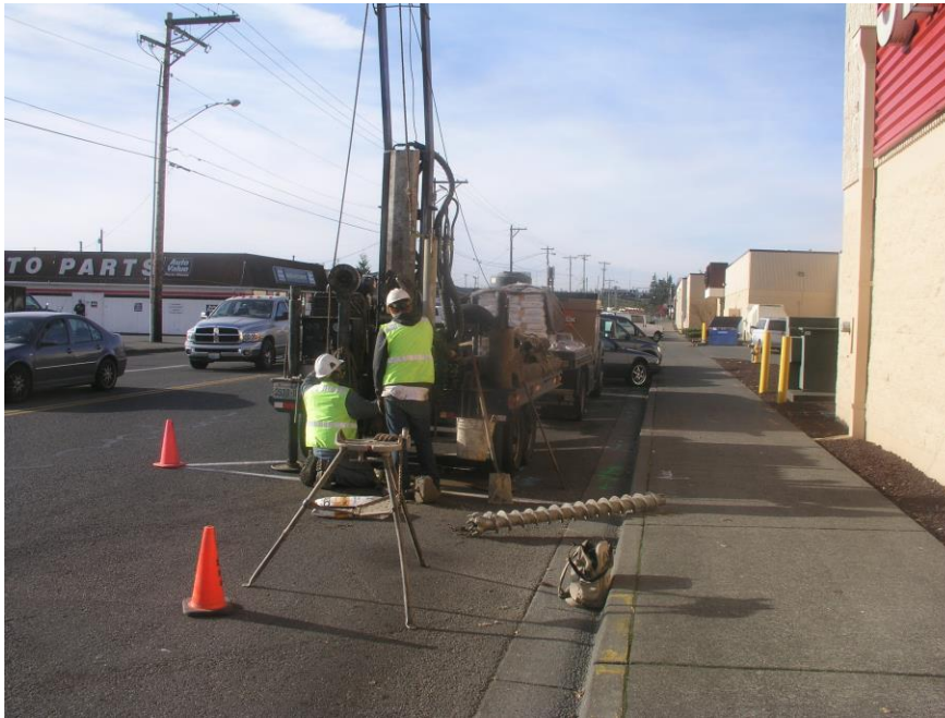
Plate 1. Looking west along 1 st Street near State Avenue. The drill rig is set up to drill boring B-3.
