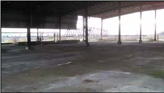
Typical interior view of the small log sawmill building on the western portion of the Subject Property.
