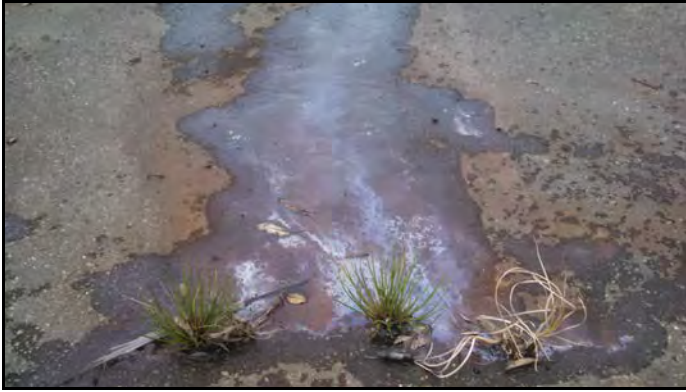
Typical view of the staining observed on the asphalt surface of the Subject Property.
