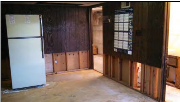
Typical interior view of the basement of the office building on the Subject Property.
