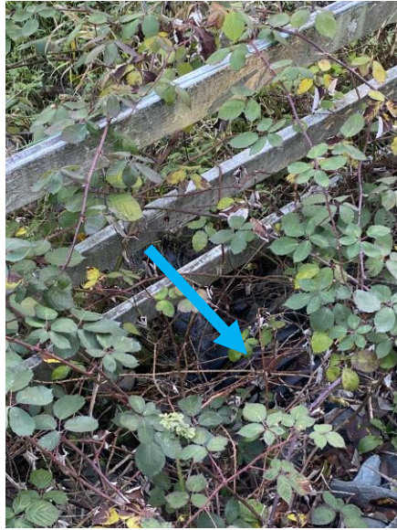
Image 9: Intersection of E Sunnyside School Rd and 83 rd Ave NE where flow crosses west under 83 rd via culvert
