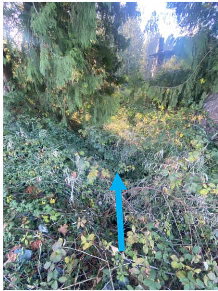
Image 10: Culvert outlet west of 83 rd where King Creek continues to quarter mile boundary
