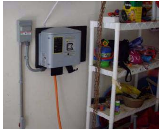
Wall-mounted Level 2 home charging station
