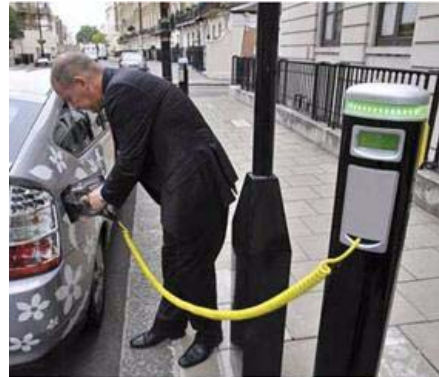
On-street charging near end of block.
