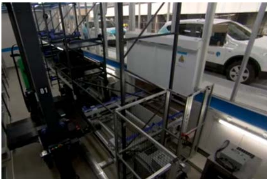
Battery Exchange Station in Tokyo
