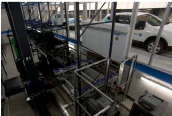
Battery Exchange Station in Tokyo
