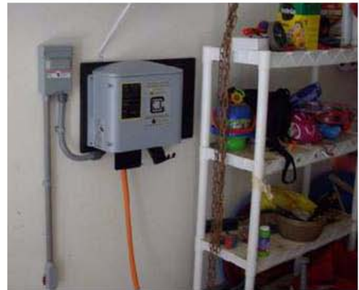
Wall-mounted Level 2 home charging station
