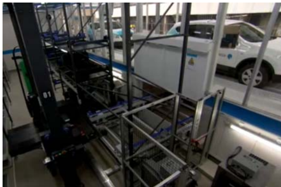
Battery Exchange Station in Tokyo
