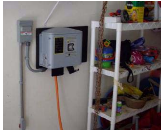
Wall-mounted Level 2 home charging station
