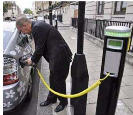
On-street charging near end of block.
