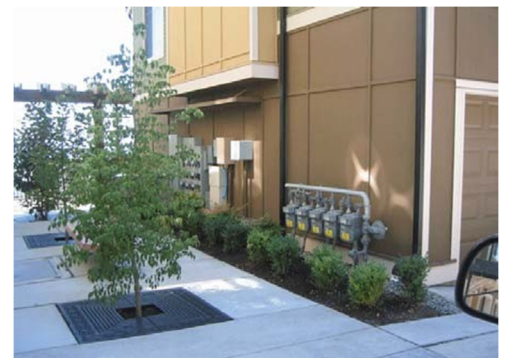
Figure 8-7. Landscaping helps to minimize the negative visual impacts of utility meters
