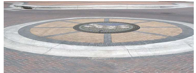
MOUNTABLE VEHICLE GRADE PAVERS (APPROX. 6"X6" CREAM/GRAY COLOR TONES) SET IN GEOMETRIC PATTERN WITH CENTER ART MEDALLION
