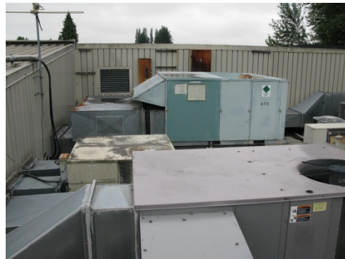
Roof Mechanical Equipment
