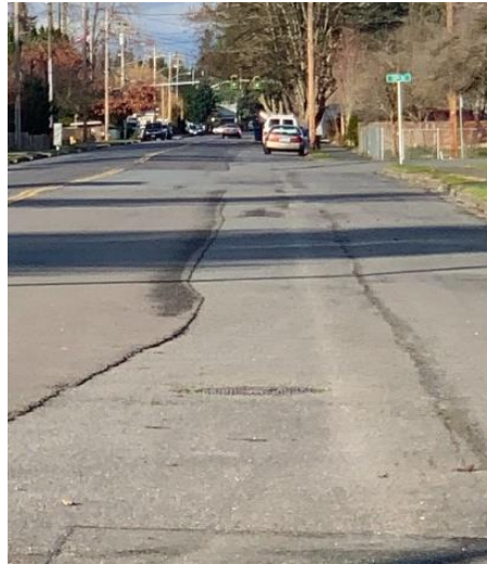
Figure 32. Quinn Ave north of 4th St
