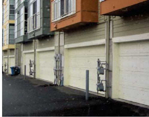
Figure B28. Exposed utility meters like this will not be allowed.
