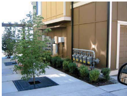
Figure B29. Landscaping helps to minimize the negative visual impacts of utility meters.
