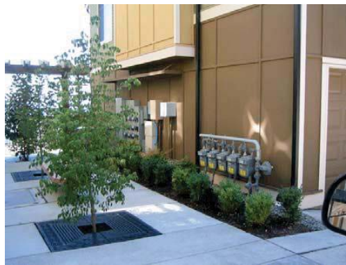
Figure C32. Landscaping helps to minimize the negative visual impacts of utility meters.
