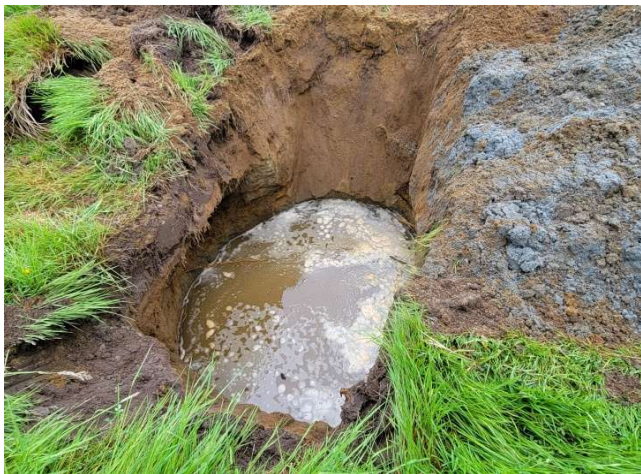
Water level began at 6 feet below surface then rose to 4 ft during excavation
