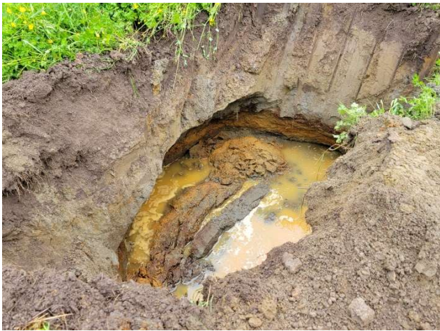
Silty materials held together in top 3 ft until further excavation caused caving.
