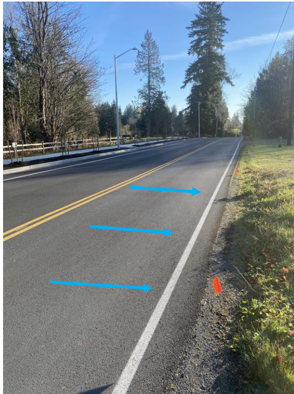
Image 3: 83 rd Ave NE frontage, contributes some upstream run-on due to lack of existing swale/ditch
