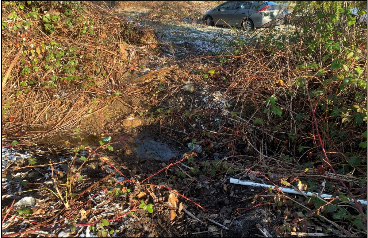
Figure 19: View northwest, drainage ditch crossing and debris on surface.
