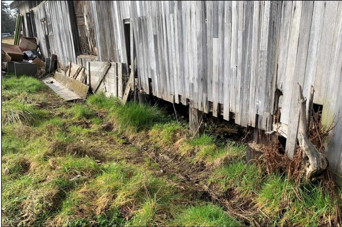
Figure 37: View southwest, Structure 1, round foundation posts visible along base of east elevation.
