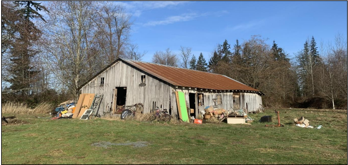
Figure 35: View northwest, Structure 1, south elevation (left), east elevation (right), and debris.
