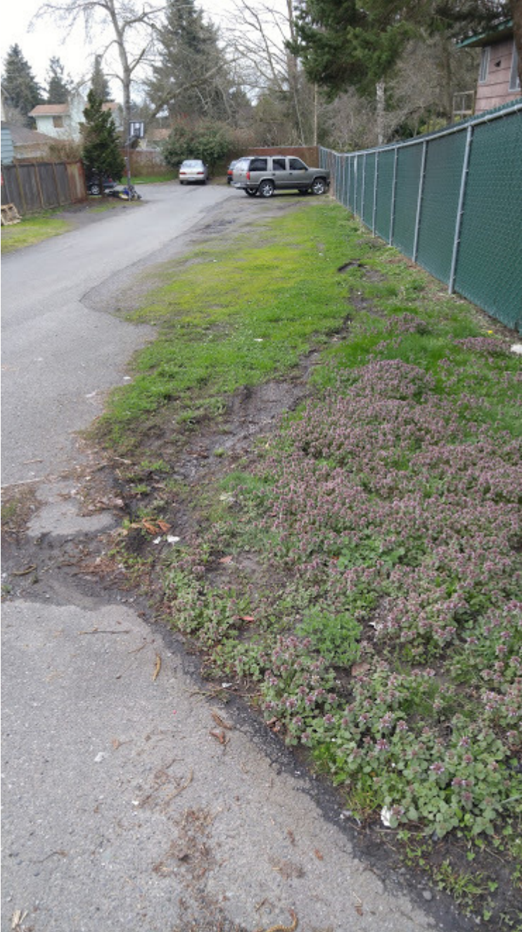
Storm water from 40 th Ave W onto site, creating scour
