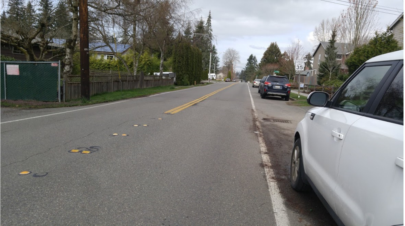
Storm water from 40 th Ave W overflows from storm drain, flows across road to corner of Jahn property, creates scour, flows to center of yard.
