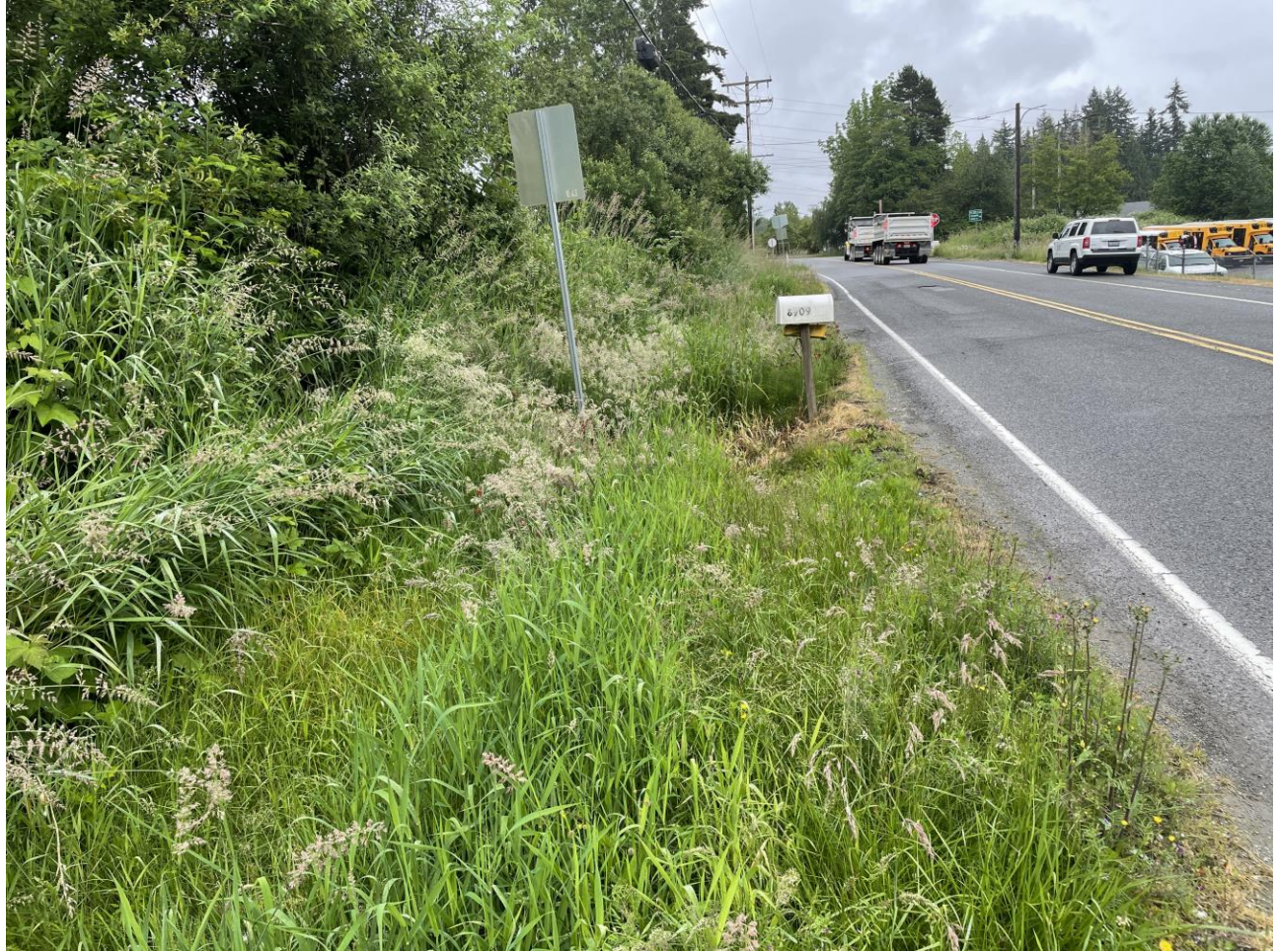
Image 6: Facing southeast at the quarter-mile boundary of analysis along the northside of Sunnyside School Road. The swale continues past the quarter-mile boundary for the downstream analysis. Per Snohomish County GIS, the swale discharges into an unnamed creek tributary to Stevens Creek.
