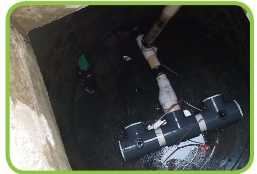
Manifold Tee View of a Cleaned System
