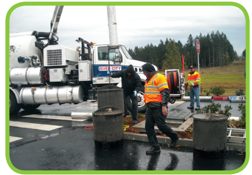
BayFilter System Cleanout
