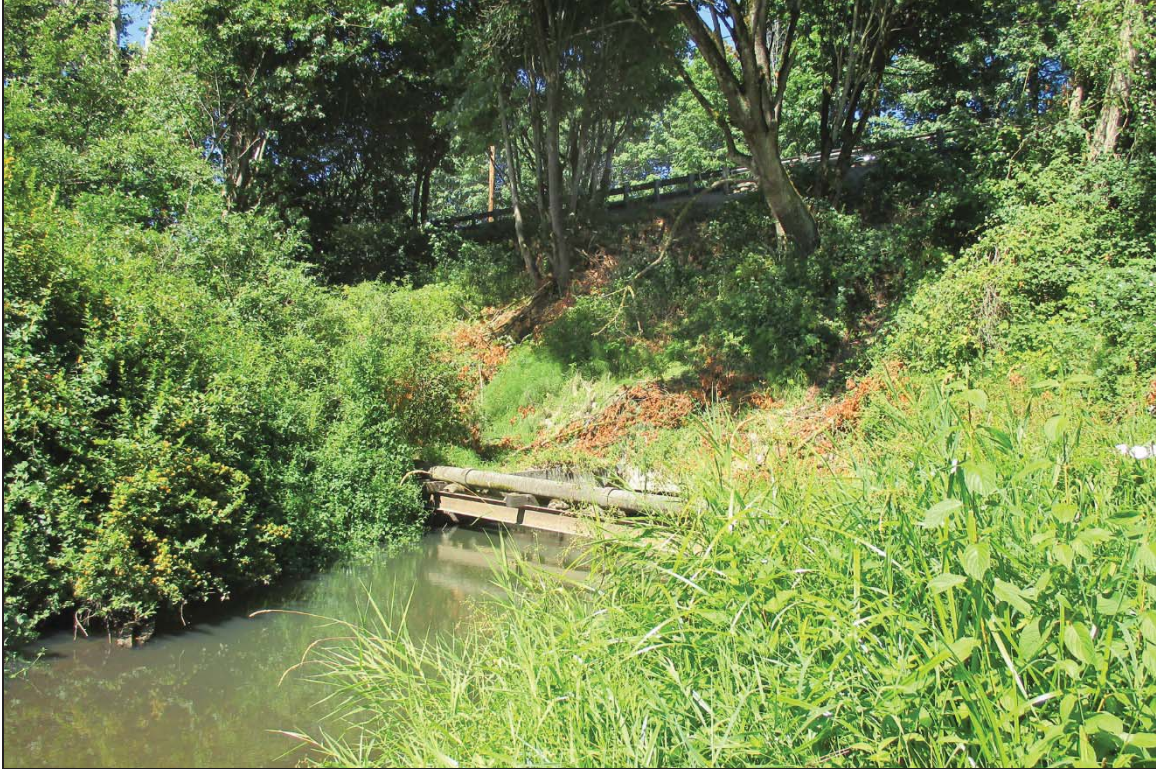
Figure 8. Existing retaining walls and utilities at the bottom of the Quilceda Creek ravine on the west side of State Avenue, view northeast.
