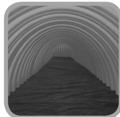
Looking down the Isolator Row from the manhole opening, woven geotextile is shown between the chamber and stone base.
