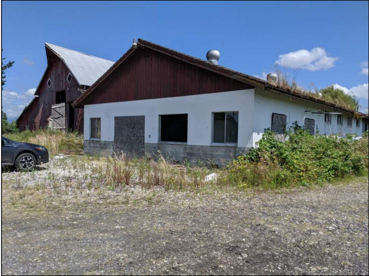
Figure 12. Outbuilding 1 (DAHP Property #722501) at 16329 51st Avenue NE. Image of west and south elevations, view to the northeast.
