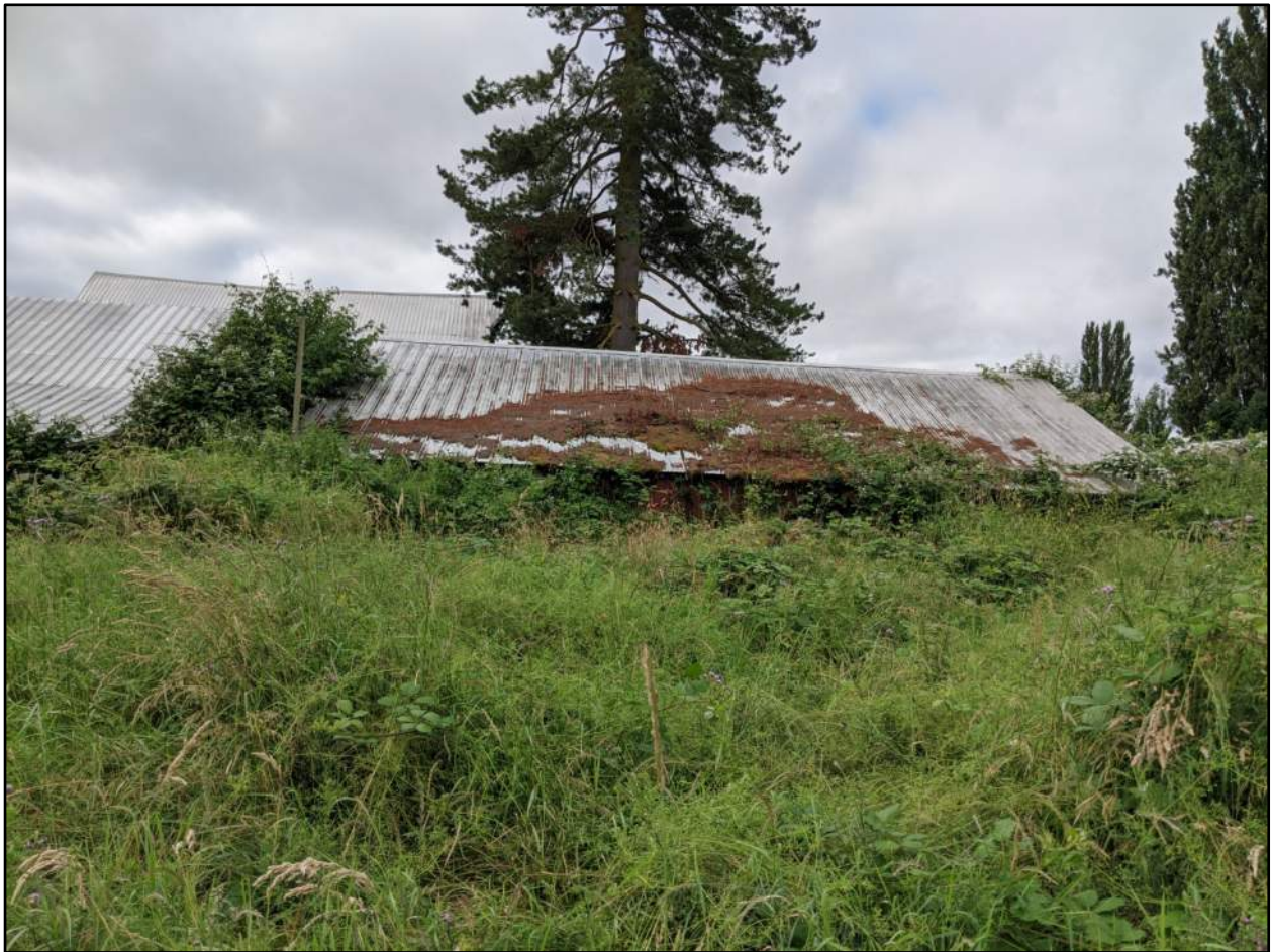
Figure 14. Outbuilding 3 (DAHP Property # 722503) at 16329 51st Avenue NE. Image of north elevation, view to the south. Trees or tall brush to left divide Outbuildings 3 and 2 (DAHP Property # 722502).
