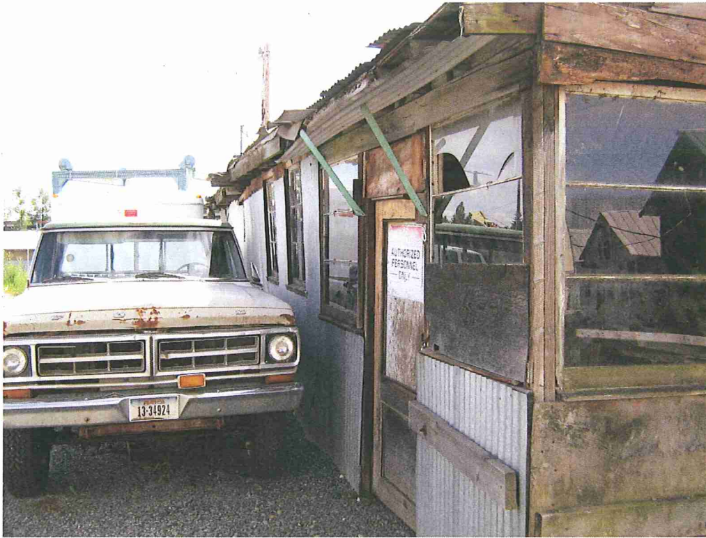
Photograph of the "prop shop" located on the southeastern portion of the subject property. Viewing to the south.
