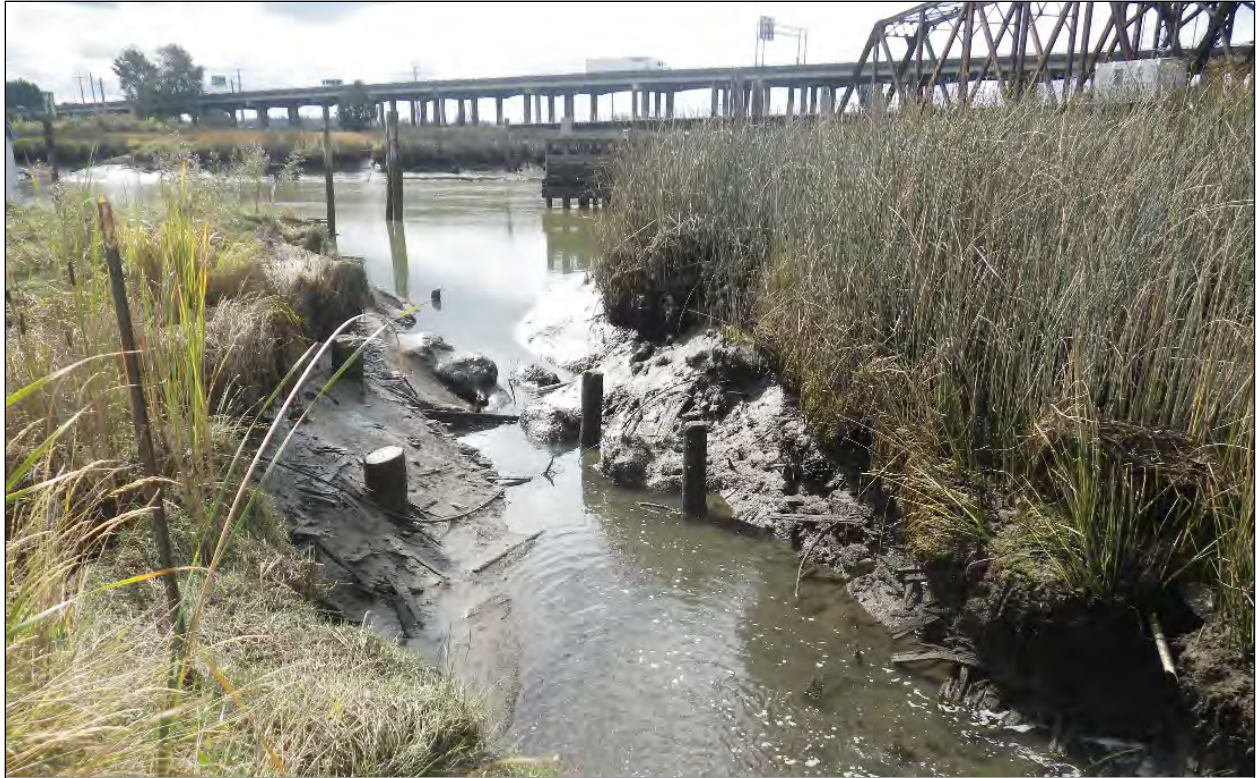
Figure 16. Piling configuration within inlet channel. View to the south from the east side of weir.
