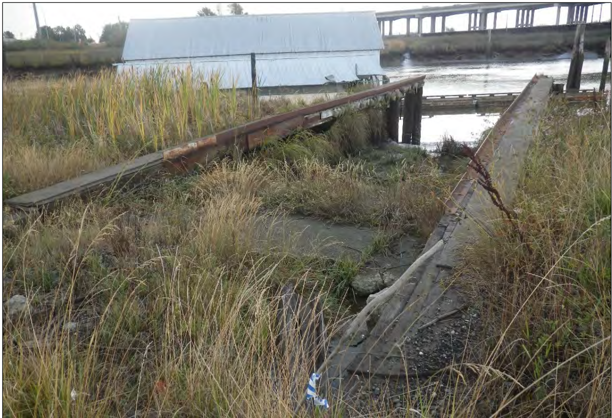
Figure 18. Boat Launch 1, extending over the Ebey Slough on pilings. View to the south.
