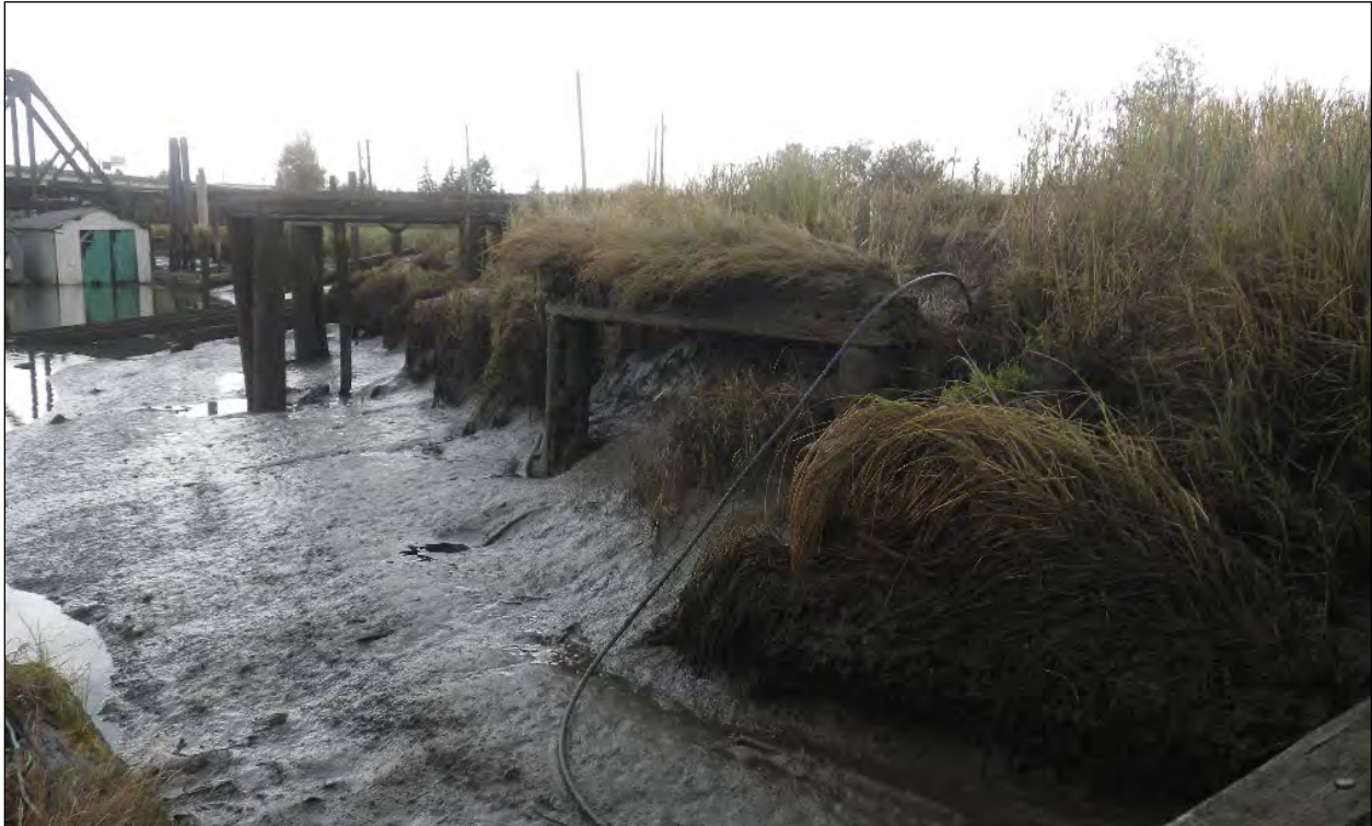
Figure 20. Two pilings and square cross-beam along embankment edge. Boat Launch 1 rails on pilings in background. View to the west-northwest.
