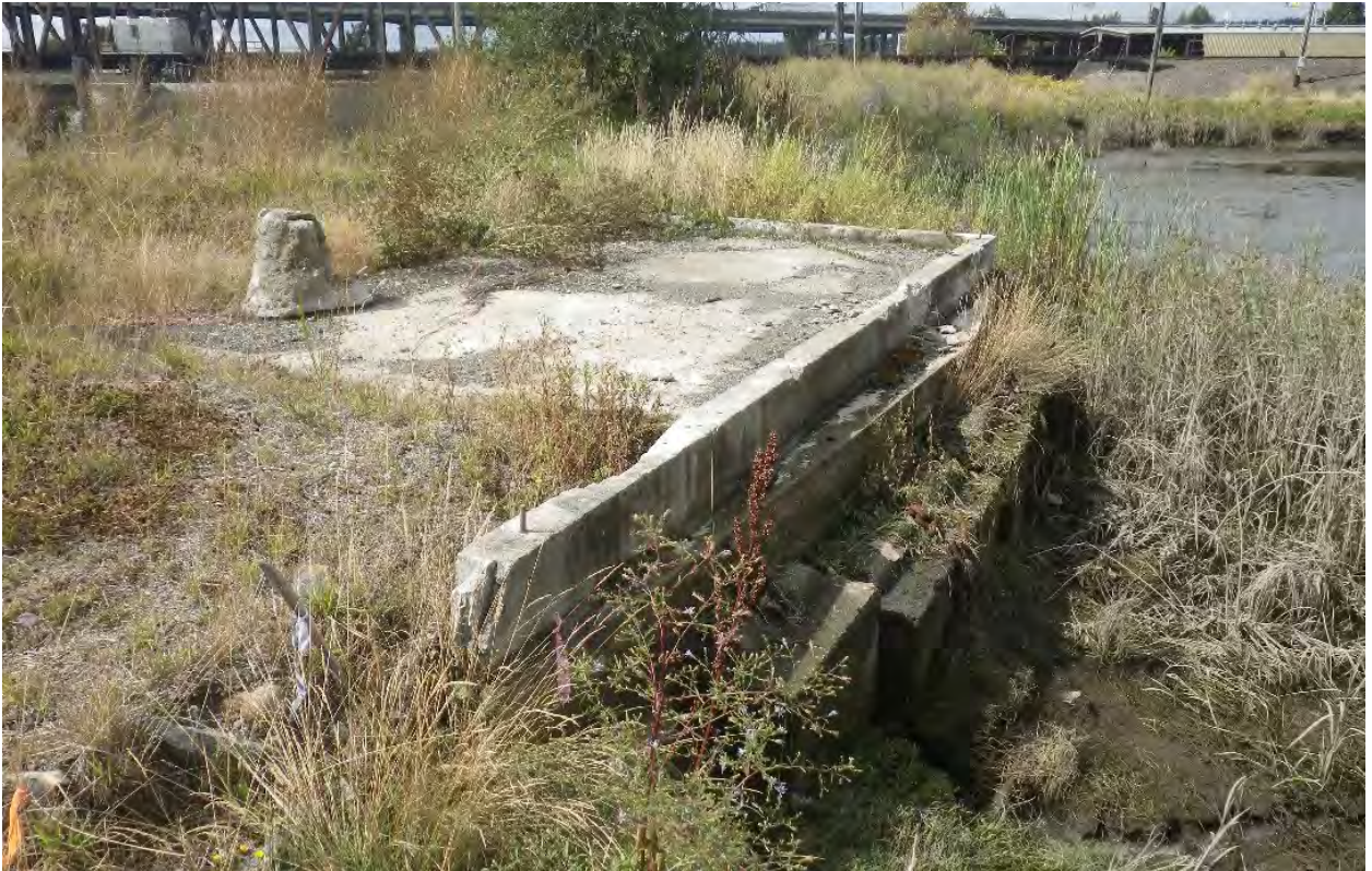
Figure 17. Concrete pad on east side of inlet. Site datum tree in background. View to the west.
