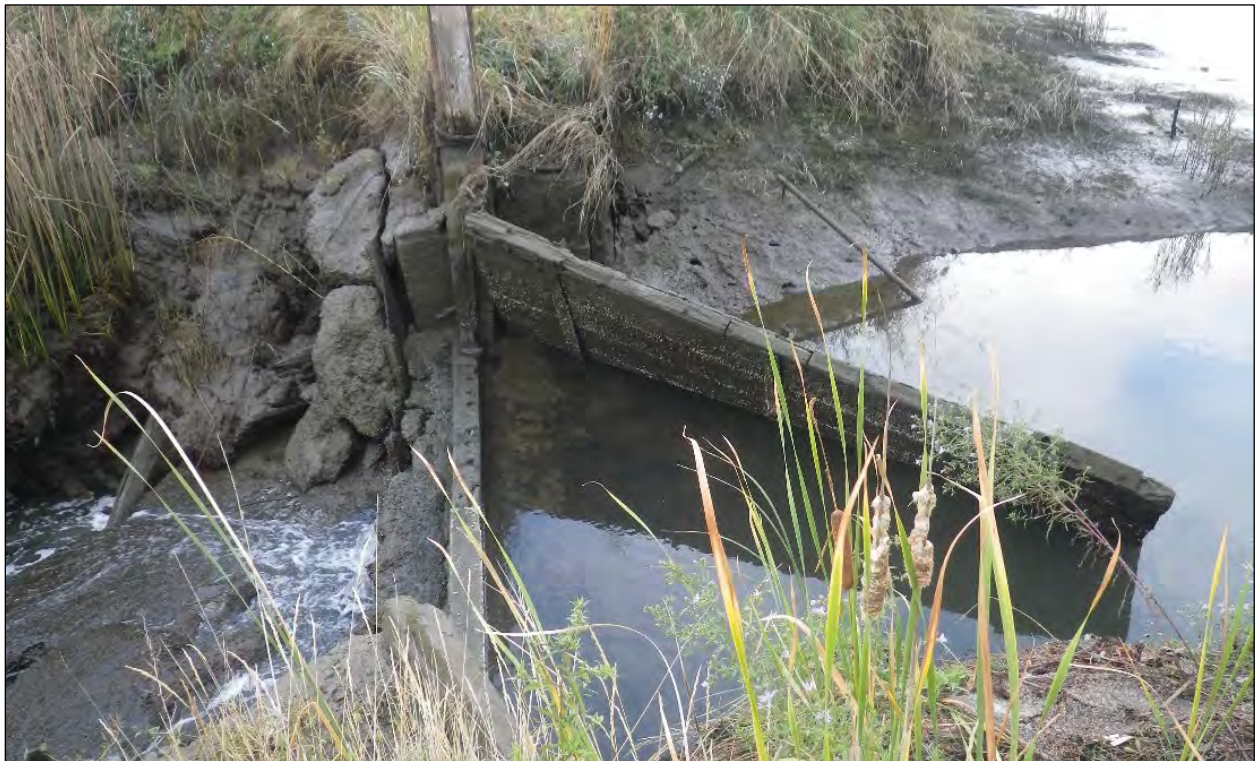
Figure 15. Weir feature. View to the west from the east side of inlet.
