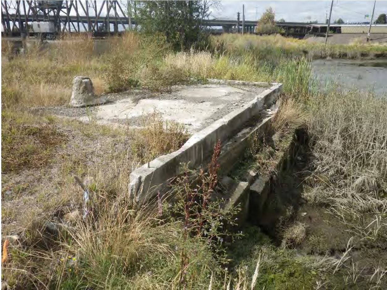
Figure 22. Concrete pad on east side of inlet and dam. Site datum tree in background. View to the west.
