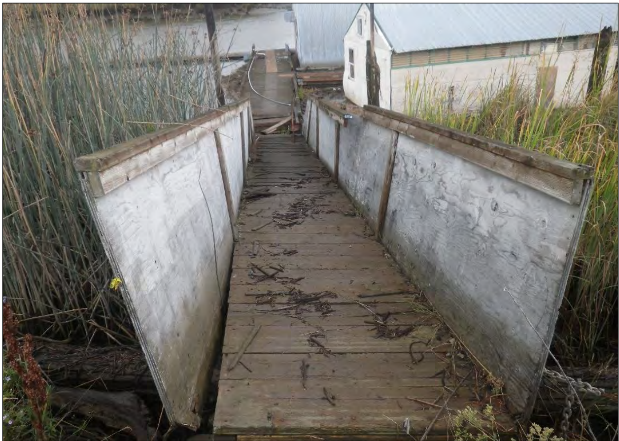
Figure 17. Ramp leading down to boathouse piers on east side of lagoon inlet. View to the south.
