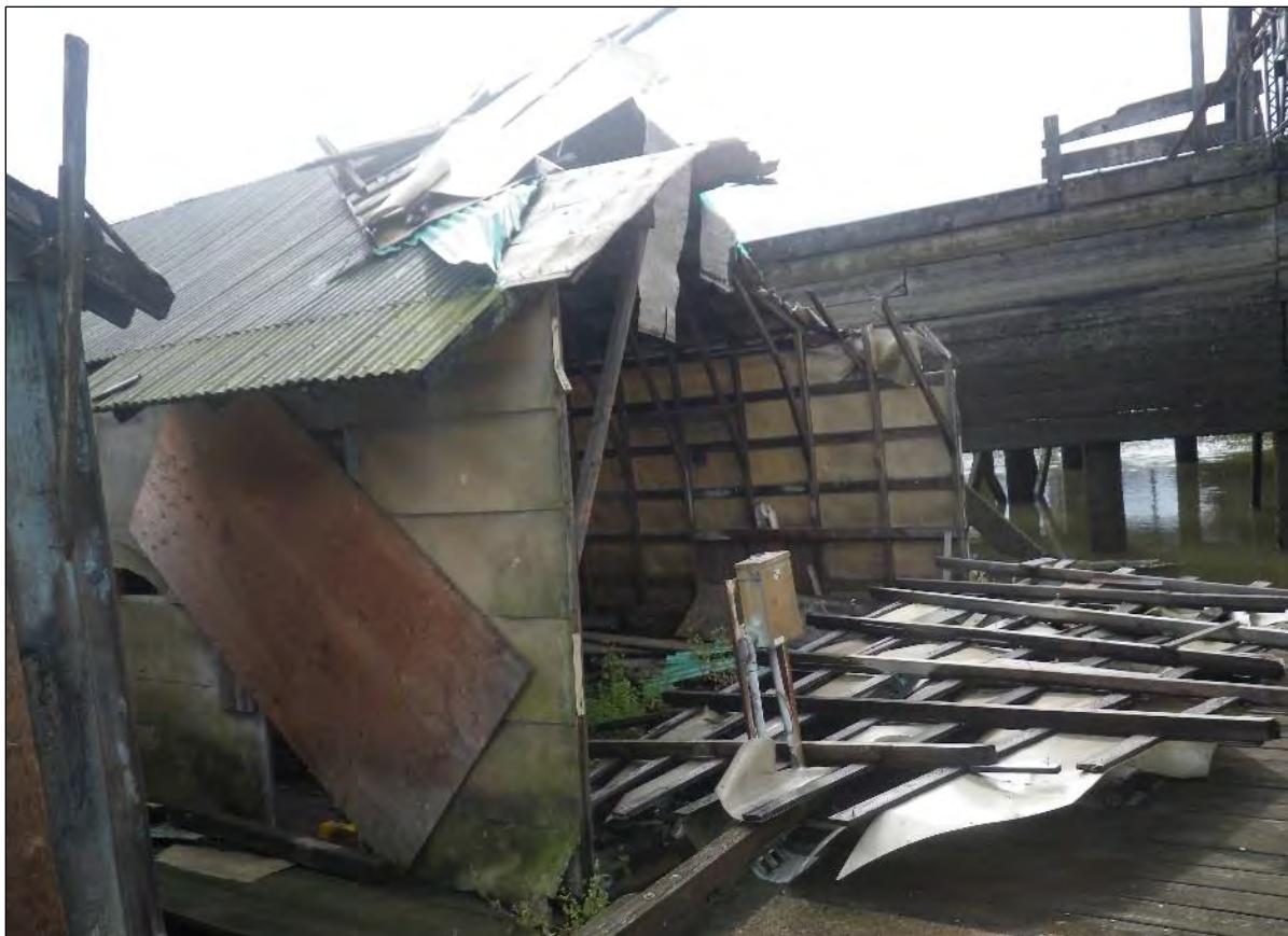
Figure 18. Boathouse shelter on west side of lagoon inlet. View to the southeast.
