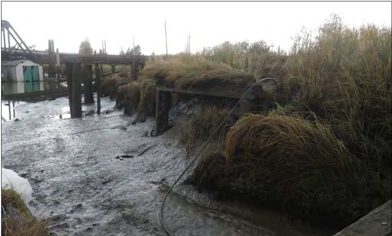
Figure 25. Two pilings and square cross-beam along embankment edge. Boat Launch 1 rails on pilings in background. View to the west-northwest.
