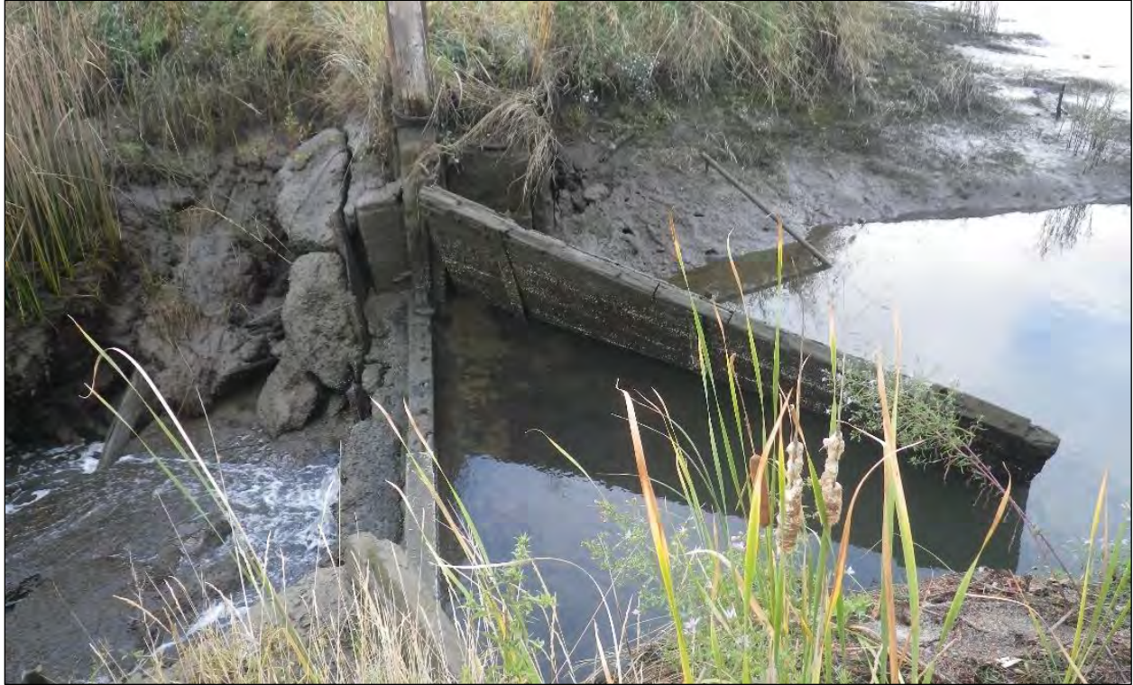
Figure 20. Dam feature. View to the west from the east side of inlet.
