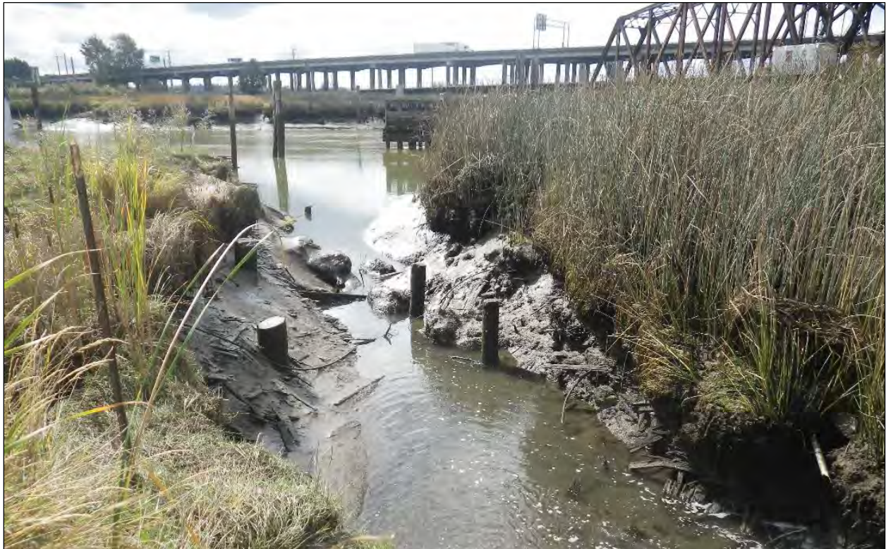
Figure 21. Piling configuration within inlet channel. View to the south from the east side of dam feature.
