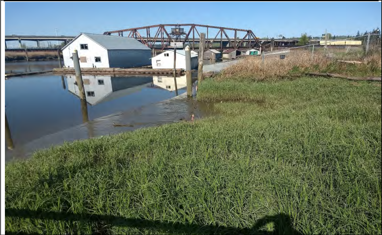
Photo 9: Unarmored portion of Wetland B along Ebey Slough looking west toward I-5 (4/25/2018). The boathouses and have since been removed. (see Photos 16 and 17).
