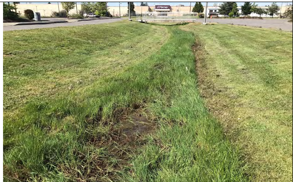
Photo 12: Constructed stormwater swale in parking area of Ebey Waterfront Park looking north toward park entrance and downtown commercial properties (4/25/2018).
