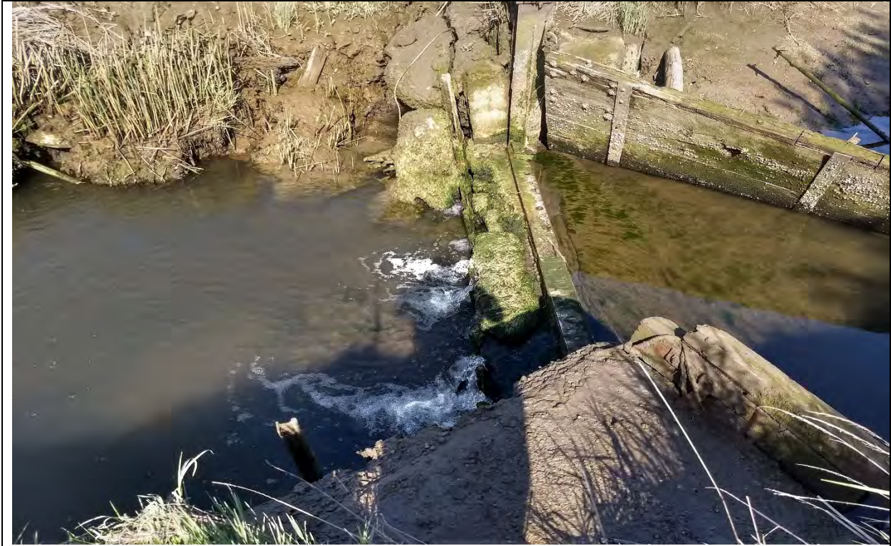
Photo 15: Dilapidated weir between lagoon and Ebey Slough. No longer functioning, so lagoon responds to tidal influence (4/25/2018).
