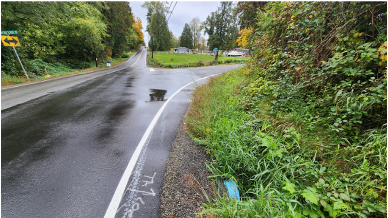
Photo 11 – Looking north at the intersection of 83 rd Avenue NE and East Sunnyside School Road. The 16-inch culvert is pictured in the bottom.
