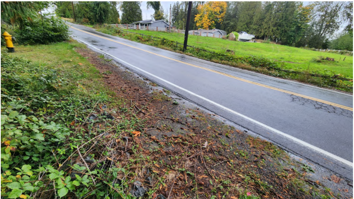
Photo 7 – Looking northeast from the west side of 83 rd Avenue NE. The outlet of the 18-inch culvert is pictured in the bottom left.
