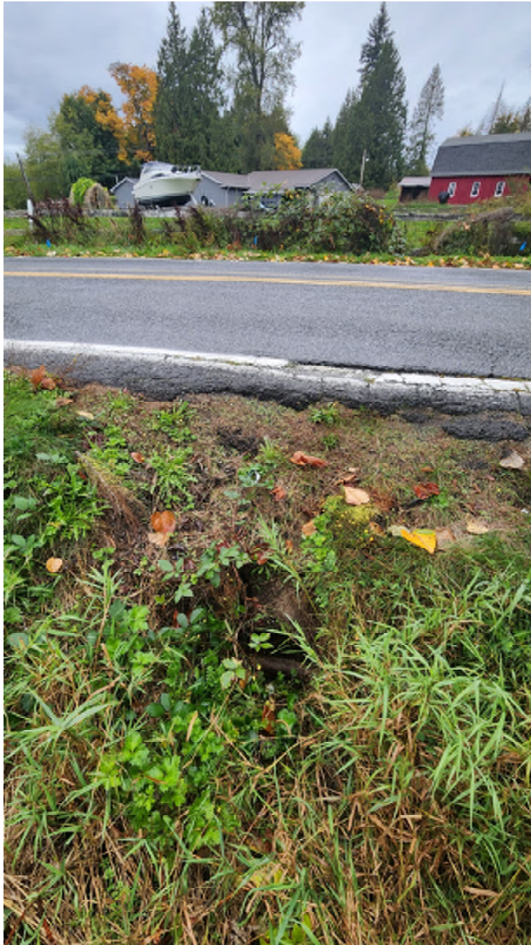
Photo 3 – Looking north along the south side of East Sunnyside School Road, picture in the bottom is the existing 15-inch CMP culvert that flows to the north underneath the roadway.
