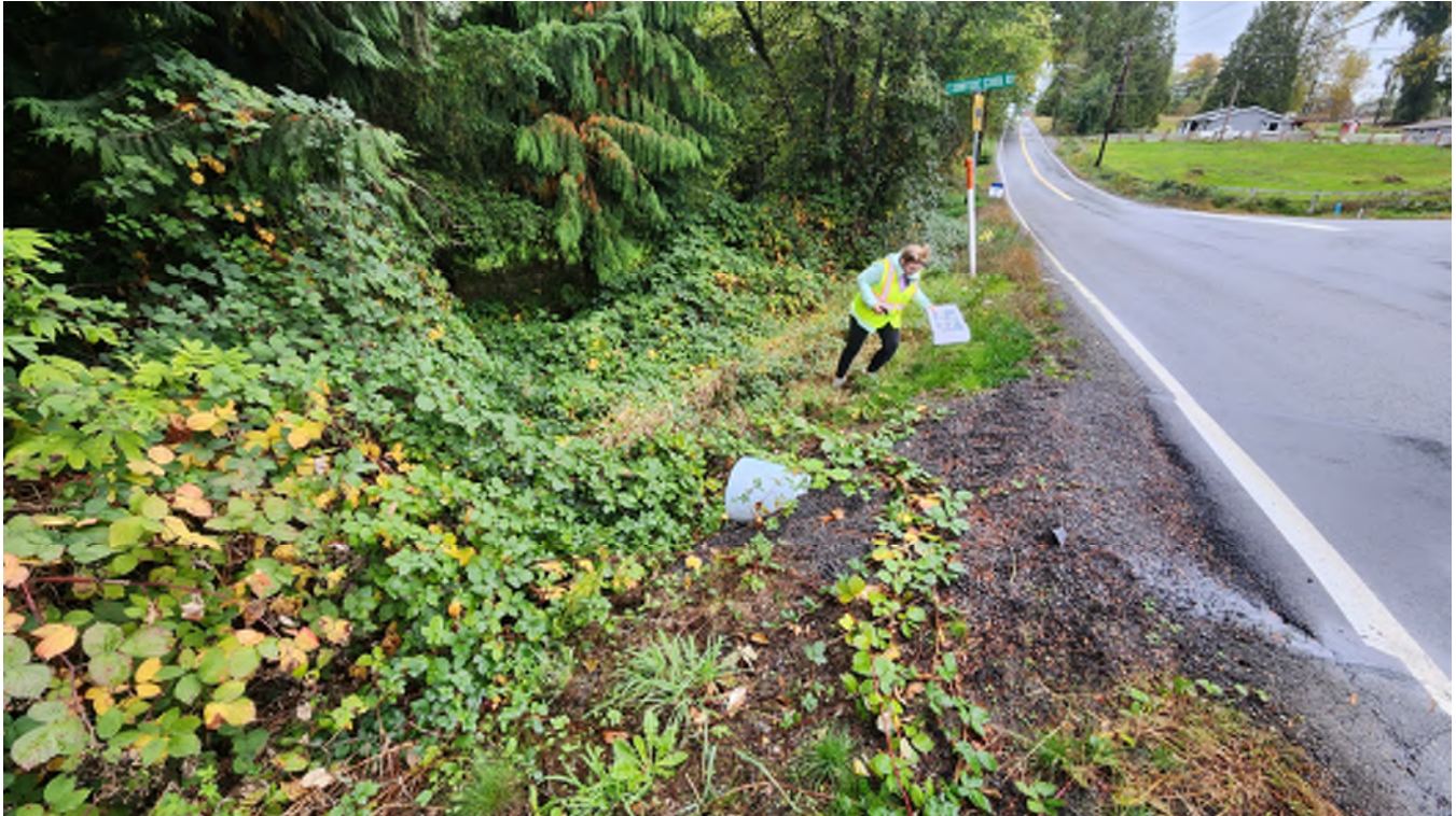
Photo 12 – Looking north along the west side of 83 rd Avenue NE at the discharge of the existing 16-inch culvert.
