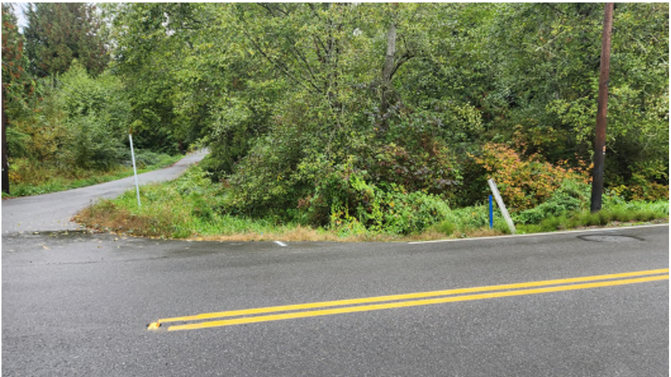
Photo 13 – Looking northwest at the intersection of 44 th Street NE and 79 th Avenue NE. The inlet to the 24-inch culvert is located near the white paint mark in the center of the picture.
