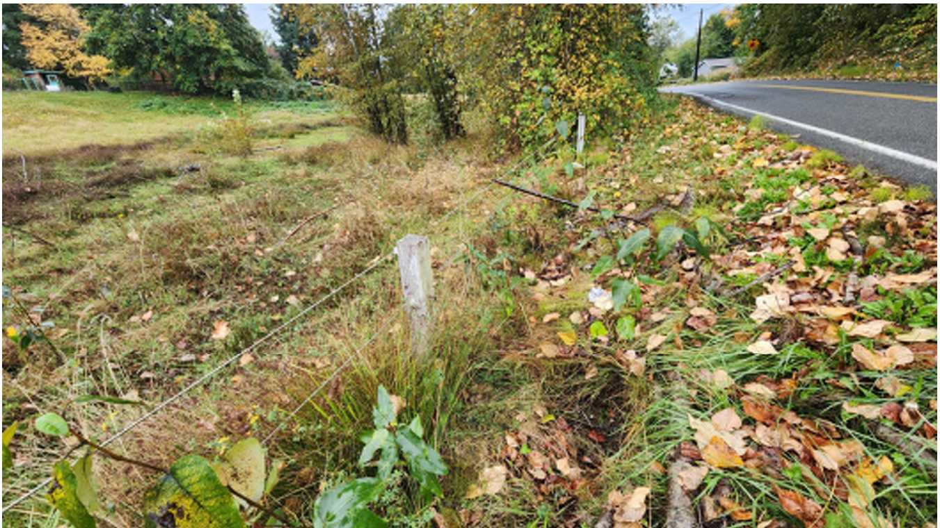
Photo 2 – Looking west along the south side of East Sunnyside School Road. The upstream culvert that discharges onto the site is pictured in the bottom and the manmade pond is pictured in the left.
