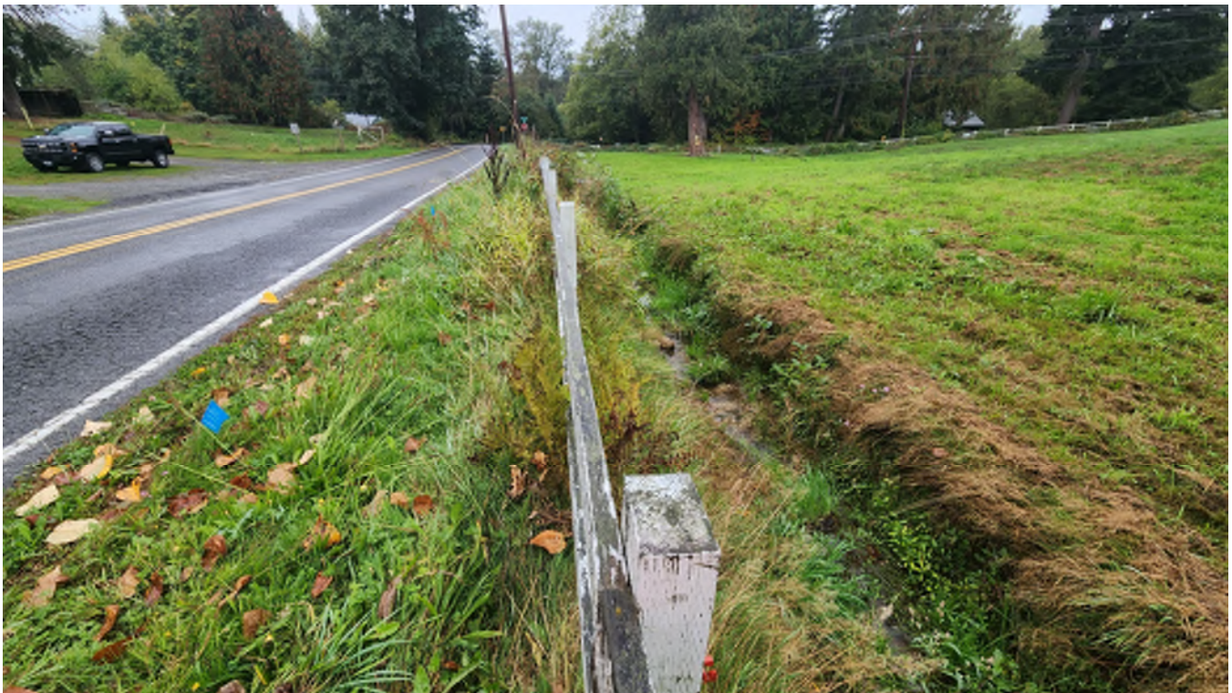
Photo 5 – Looking southwest along the north side of East Sunnyside School Road at the existing ditch that continues to the west to 83 rd Avenue NE
