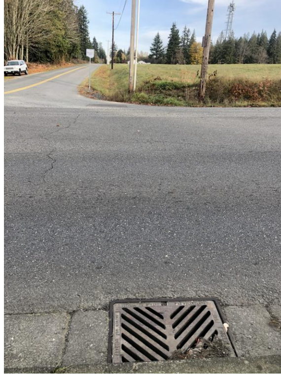
Image 2: Facing northward from the southern edge of Soper Hill Road, at its intersection with 87 th Ave NE. Discharged flows enter the existing Soper Hill collection and conveyance system on the southern edge of the road, and convey westward through closed pipe beyond the 0.25-mile boundary of analysis.
