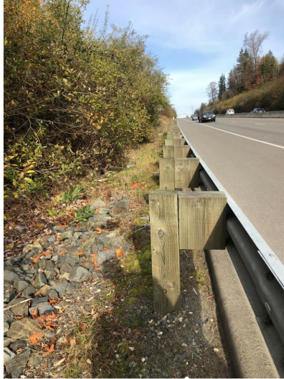
Image 6: Facing northward from the western edge of Highway 9. Discharged flows are conveyed to the existing Highway 9 collection and conveyance system and continue southward within that system until crossing beyond the 0.25-mile boundary of analysis.
