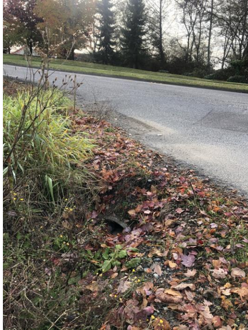
Image ❶: Facing southward from the southwestern corner of the White Barn Commercial property, at the intersection of Soper Hill Road and 87 th Ave NE. Flows discharging from Threshold Basin A flow southward through a 12" CMP culvert across Soper Hill Road and enter the existing Soper Hill collection and conveyance system.
