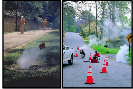
Digital Photograph Examples of smoke exit locations
