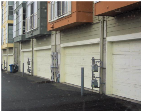
Figure C31. Exposed utility meters like this will not be allowed.
