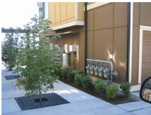
Figure C32. Landscaping helps to minimize the negative visual impacts of utility meters.
