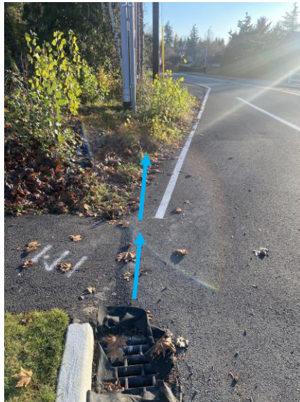
Image 4: storm conveyance system continues south along 83 rd Ave
