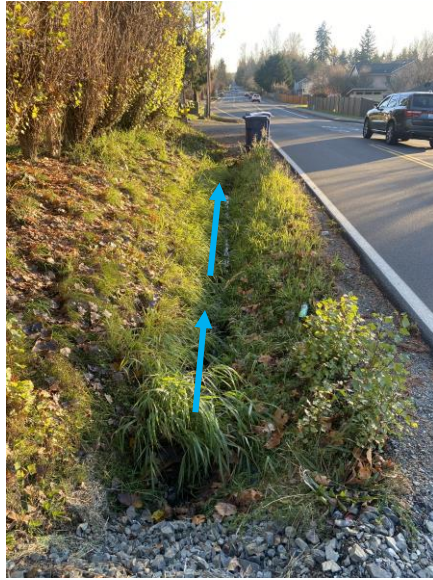
Image 5: Closed conveyance pipe outlets into grass swale along 83 rd Ave
