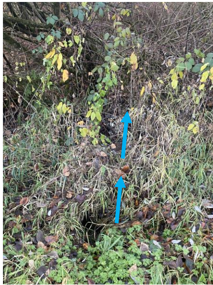
Image 10: Culvert outlets to wetland area on south side of Soper Hill Rd, continues beyond quarter mile boundary
