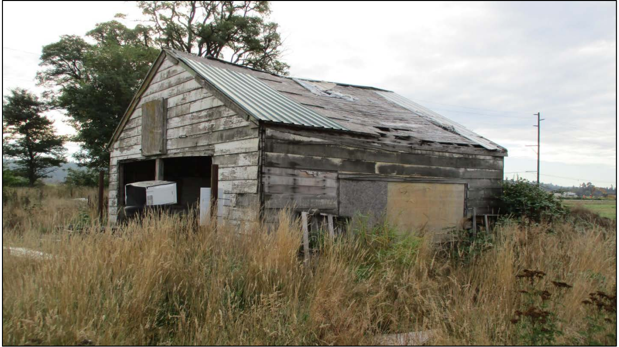
Figure 8. Deteriorated garage present at the eastern margin of the property at 16204 51 st Avenue NE.
