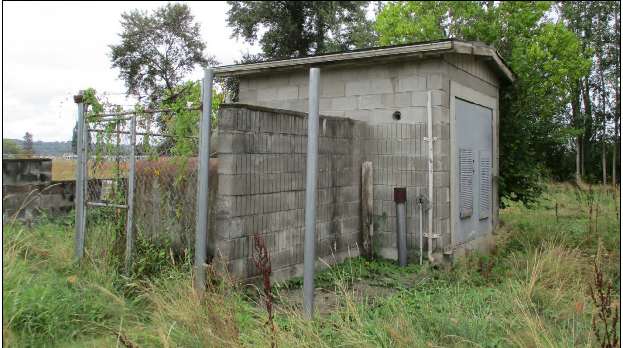
Figure 7. Concrete block structure located at the southeast corner of the property at 16430 51 st Avenue NE. View to southeast.
