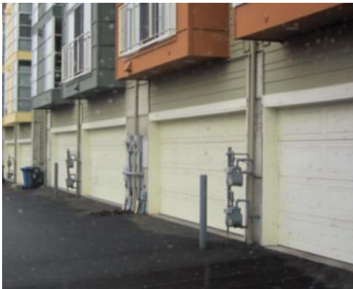
Figure 24 – Exposed utility meters like this will not be allowed
