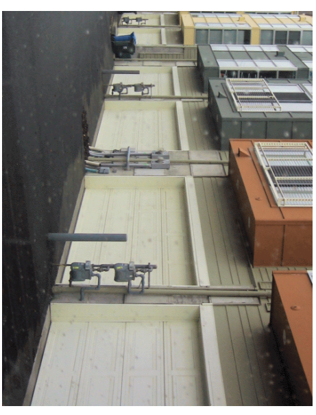
Figure F-6. Exposed utility meters like this will not be allowed.
